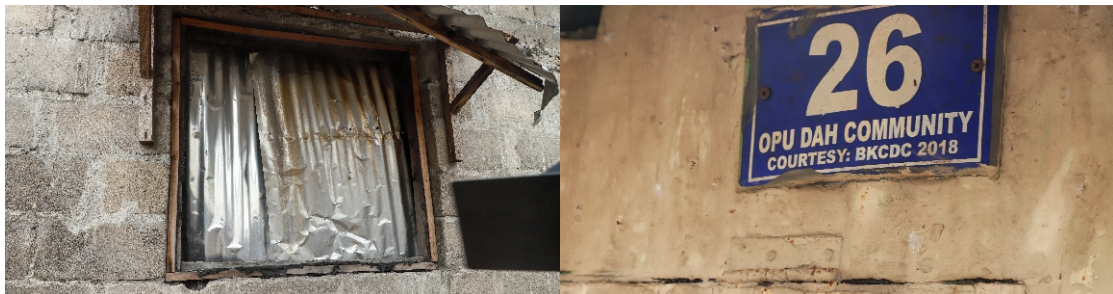
Scorch marks on a window at 26 Opu Dah Compound following a fire linked by residents to gas escaping from a nearby borehole
